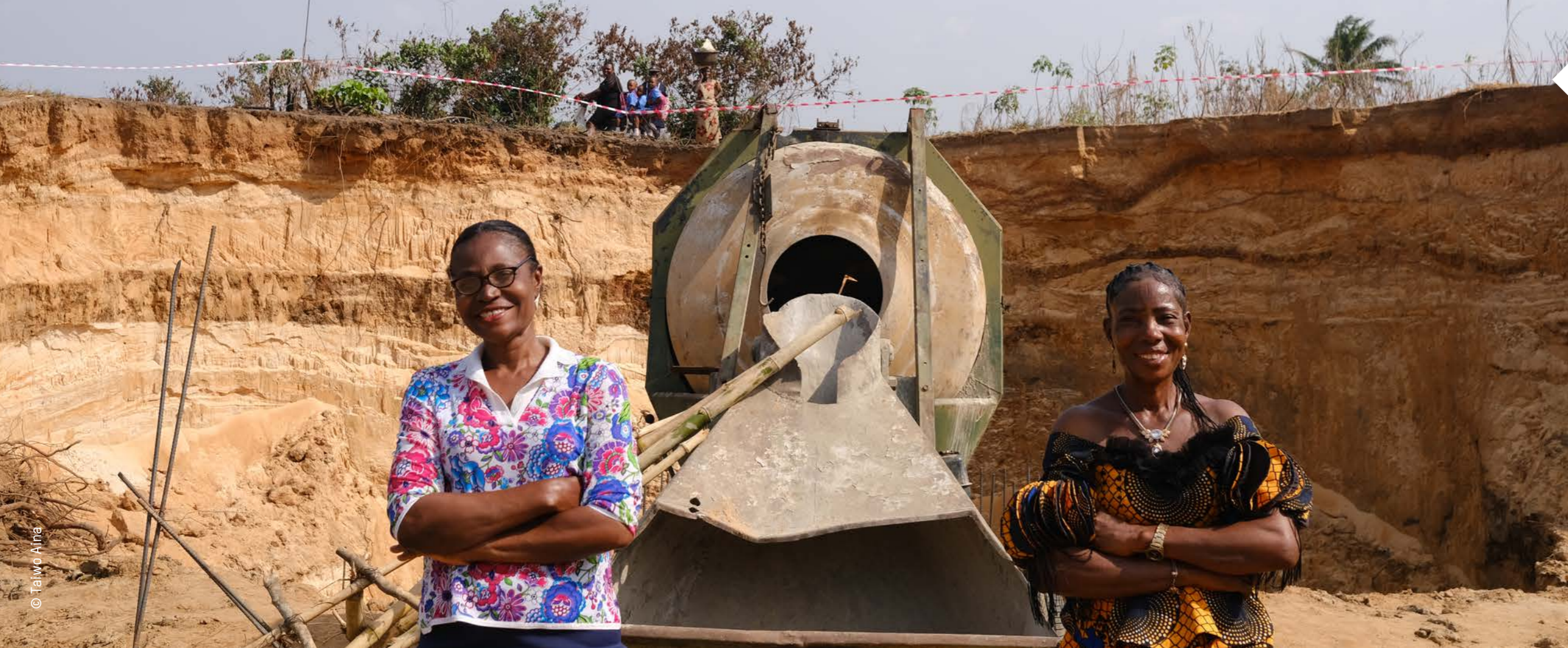
Virginia Obianyo from CISLAC and a female leader standing at the construction site of the bridge they lobbied for with the local government in Enugu State, Nigeria.
