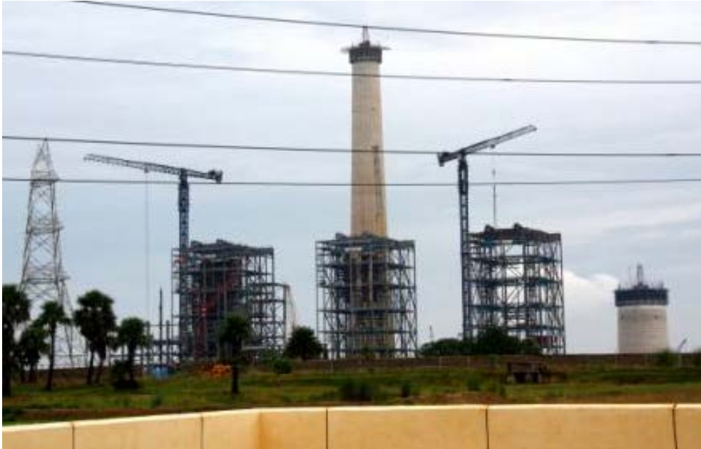
The GKEL power plant in Odisha. Photo: Joe Athialy
